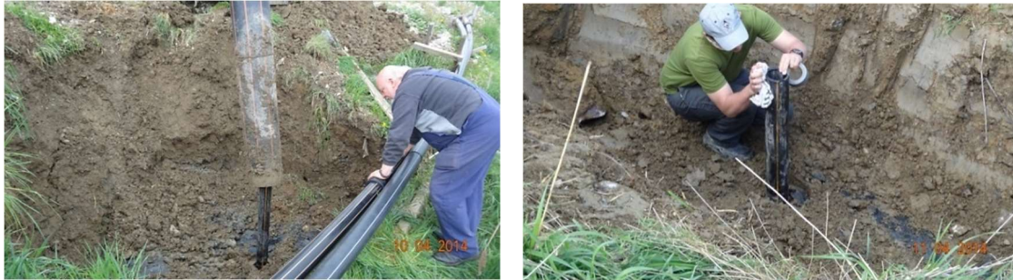
Fig. 17.7 a+b Opening and preparing a well head for measurement
