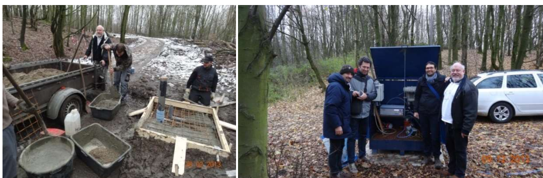
Fig.17.14 a+b Preparing the area for the container with the test equipment and the container with guests from Italy
