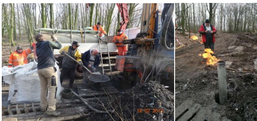
Fig.17.13 a+b Filling the drill hole with cement suspension and the flame from the landfill gas on top of the pipe
